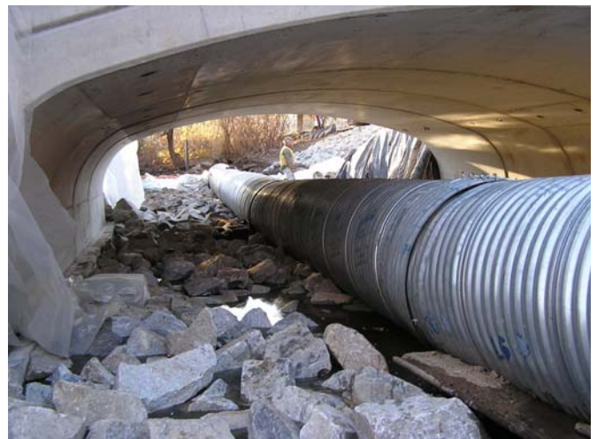
View underneath new bridge structure with stream bypass pipe still in place (above)
