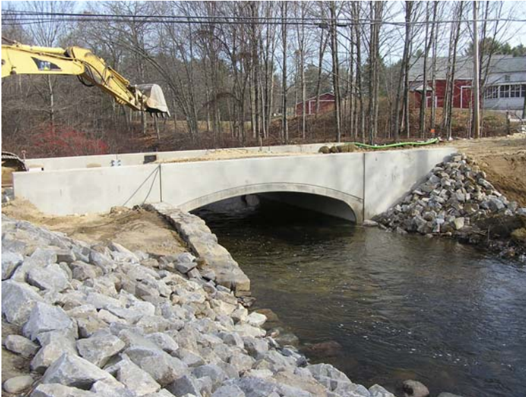
At Left Looking Upstream at New Bridge: Restoration of natural stream flow; diversion pipe removed and stone protection in place.
